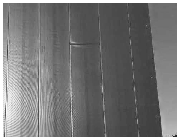
Picture n° 2: deformed wall
